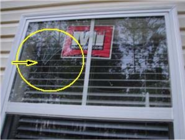
G. Picture 1 Broken window - rear side of home.
